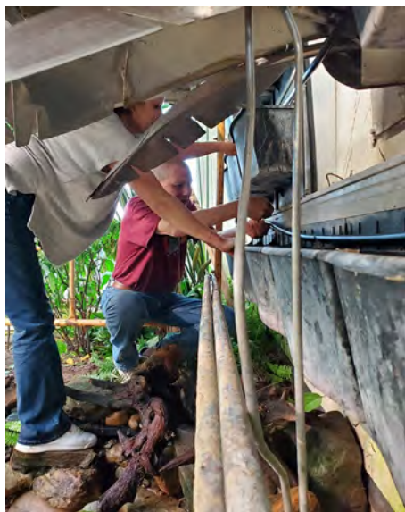
Jody Davey and Paul Fedyk install a new irrigation system so the plants can more easily receive the nutrients they need to grow.
